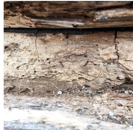
Dry rot and powder post beetle damage
